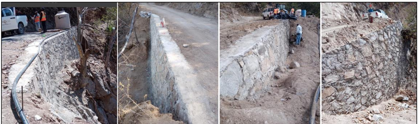
Figure 4-3: Access Road Stability Retaining Walls Built by Community Members with Oroco Financial Support
